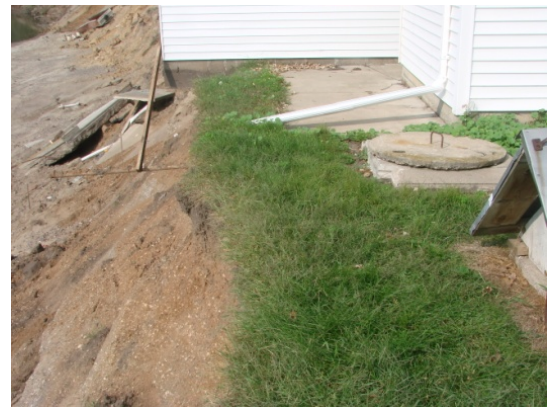
Washed away SSTS in eroded stream bank
